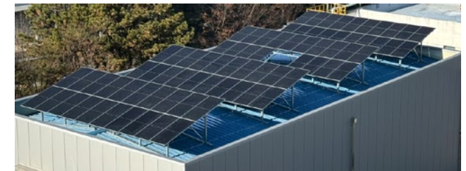
Cheonan Campus Solar Power Generation Facilities
